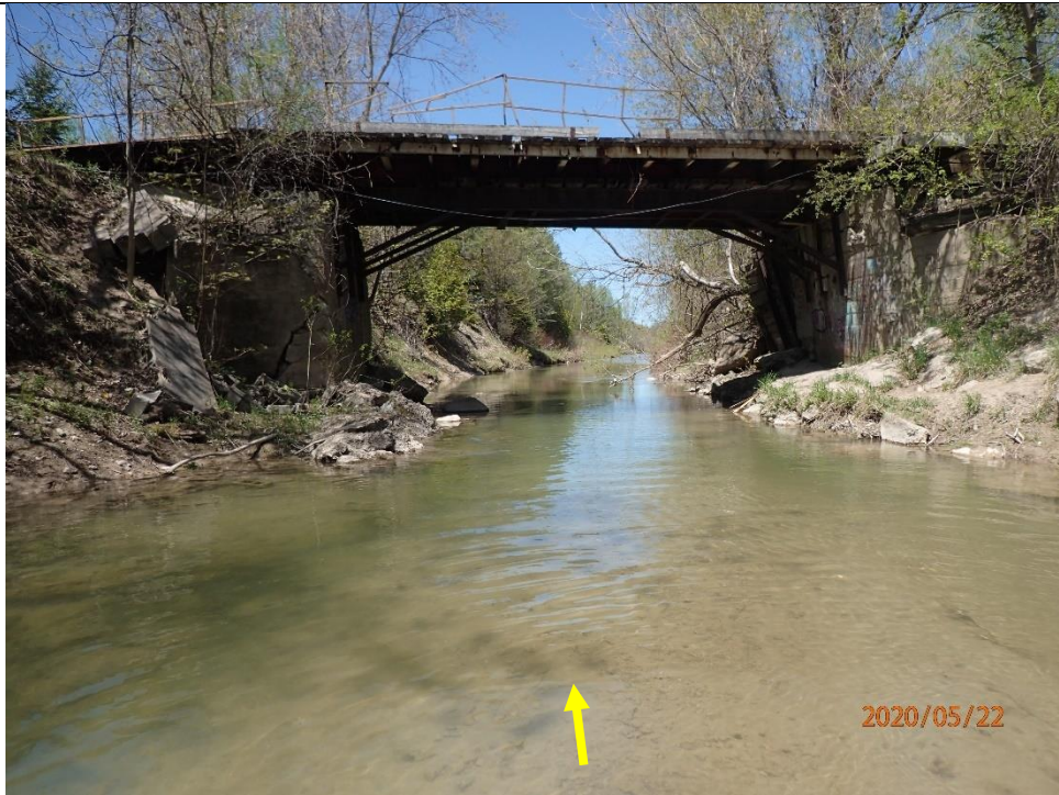
Photograph taken at the downstream extent of the reach where a driveway bridge crosses the watercourse. Bankfull width and depth were 11.54 m and 0.76 m, respectively.
