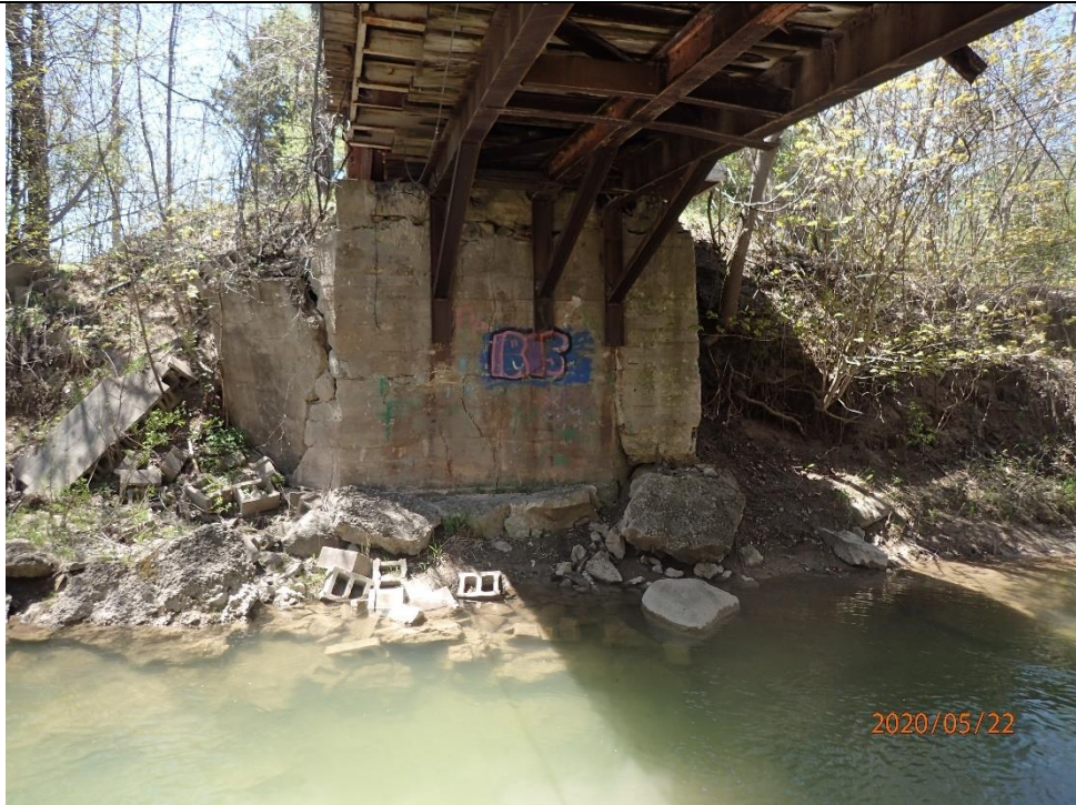
Photograph looking at the exposed and worn concrete bridge footings associated with the driveway crossing. This provides evidence of degradation, which limits overall channel stability.
