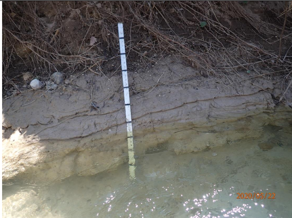
Photograph taken of the right bank showing exposed till. The channel was worn into undisturbed overburden / bedrock this is indicative of degradation.
