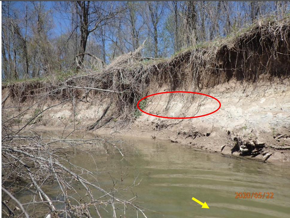
Photograph taken facing upstream. The channel had unstable slopes and bank failures were observed frequently. Suspended armour layer was visible (circled here) throughout the reach.
